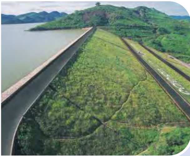
Podagada Earthen Dam in Orissa is 462mts in length and 72 mts in height. The dam was completed in 1996.
