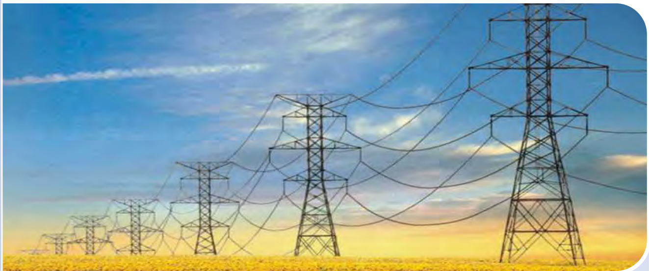
Power Transmission and Distribution
