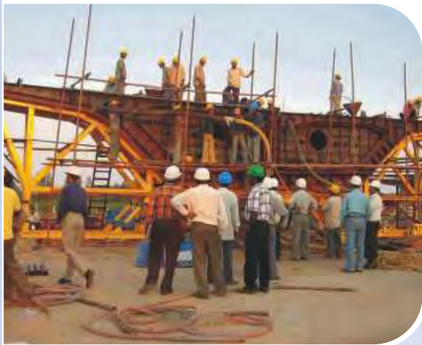
Work in full swing at Bangalore Elevated Highway Project. The 10 km Expressway to ease the traffic problem on Bangalore-Hosur road.
