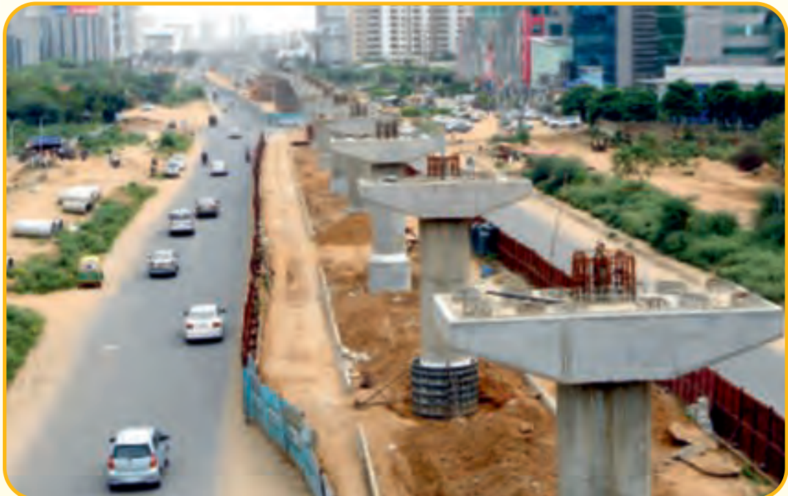
Rapid Metro Rail Gurgaon (RMRG) Phase-II Viaduct Crash Barrier & Pedestal work in progress (with completed Piers/Pier Caps)
