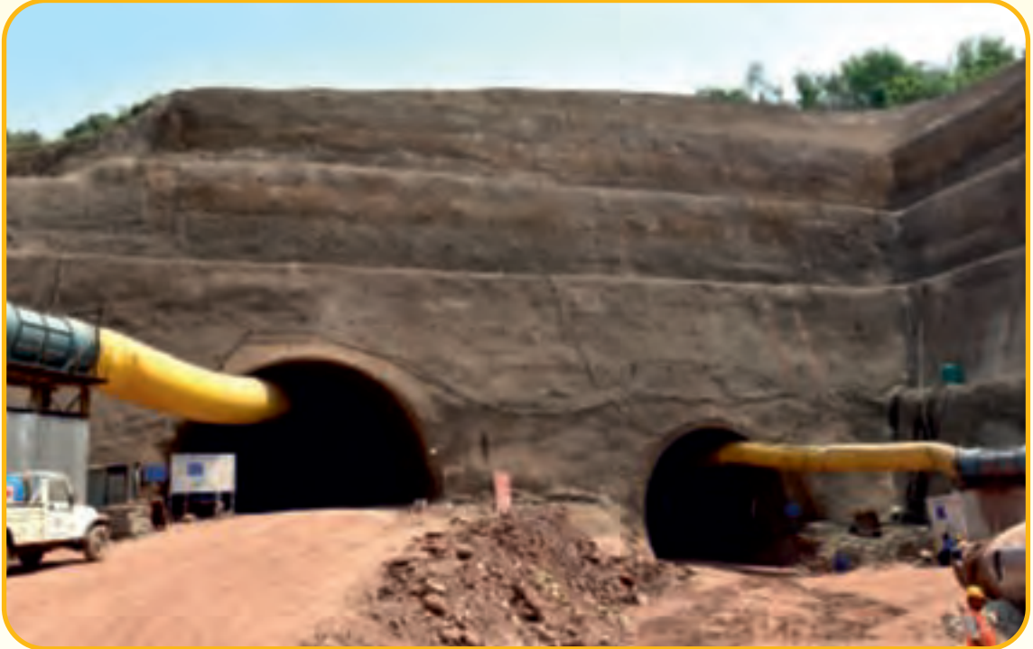
Construction of Main Tunnel and Escape Tunnel work in progress at Kiratpur – Ner Chowk Road Project, Himachal Pradesh
