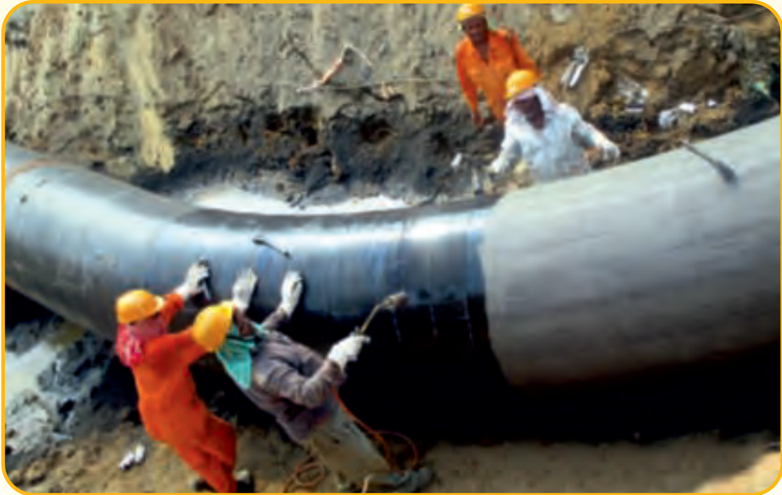
48" Pipeline - Coating of Hot Bend Pipe at Mangalore Padur Pipeline Project for Indian Strategic Petroleum Reserves Limited (ISPRL), Ministry of Petroleum and Natural Gas, Government of India
