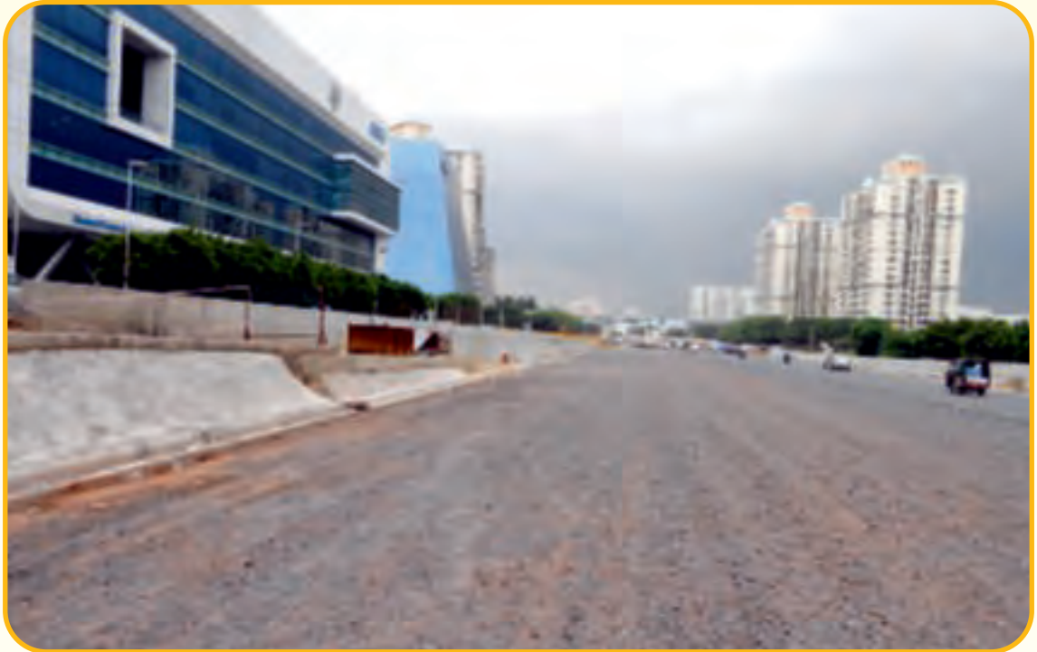
Dense Bituminous Macadam (DBM) layer completed at Cyber City area at DLF Road Project, Gurgaon
