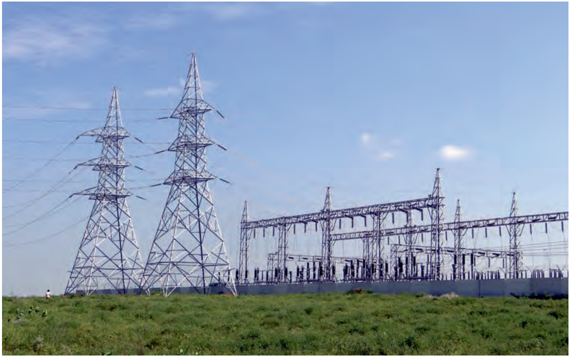
132 kV Switch Yard at Machraulli, Jhajjar, Haryana
