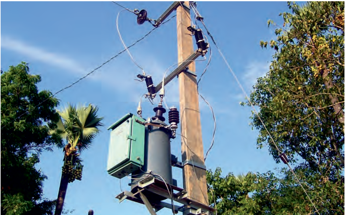
Pole Mounted 10kVA Transformer Inside a Village for Below Poverty Line (BPL) Consumers of Sundergarh District, Odisha (Rural Electrification Works)
