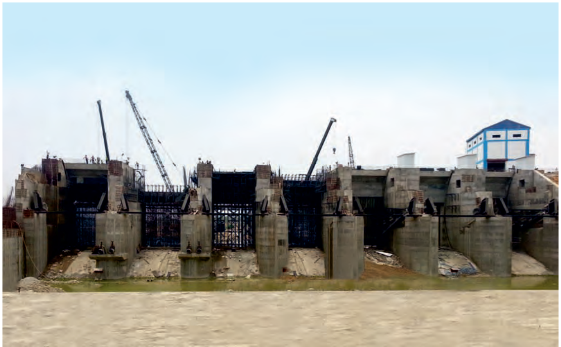
Down Stream View of Anuppur Barrage Project at Son River, Anuppur District, Madhya Pradesh
