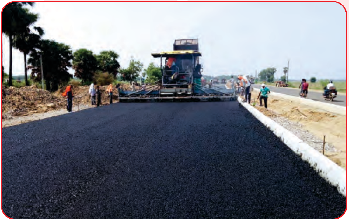
Four Laning of Patna Gaya Dobhi Section of NH-83 Road Project, Bihar
