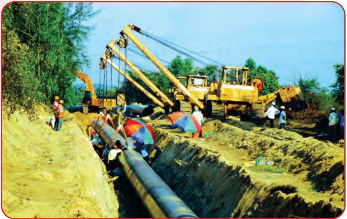
EPC Pipeline Laying Project in Karnataka for Indian Strategic Petroleum Reserves Limited (ISPRL), Ministry of Petroleum and Natural Gas, Government of India
