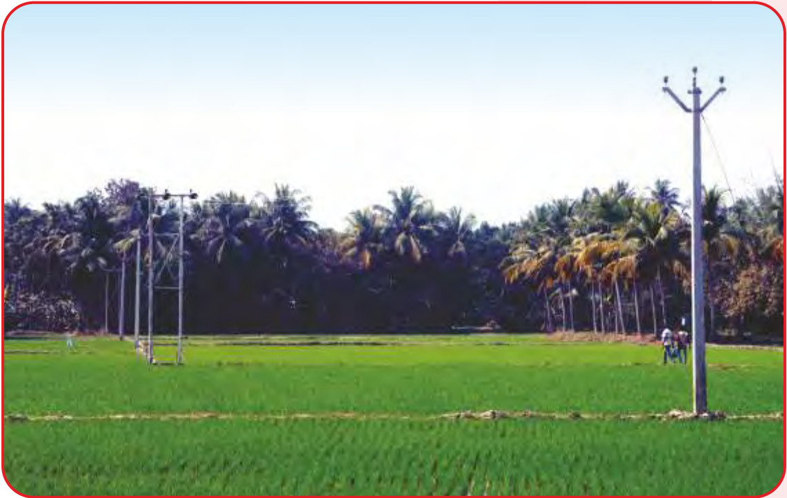
RE Works for West Bengal State Electricity Distribution Company Limited (WBSEDCL) in 24- Paraganas (South) District, West Bengal
