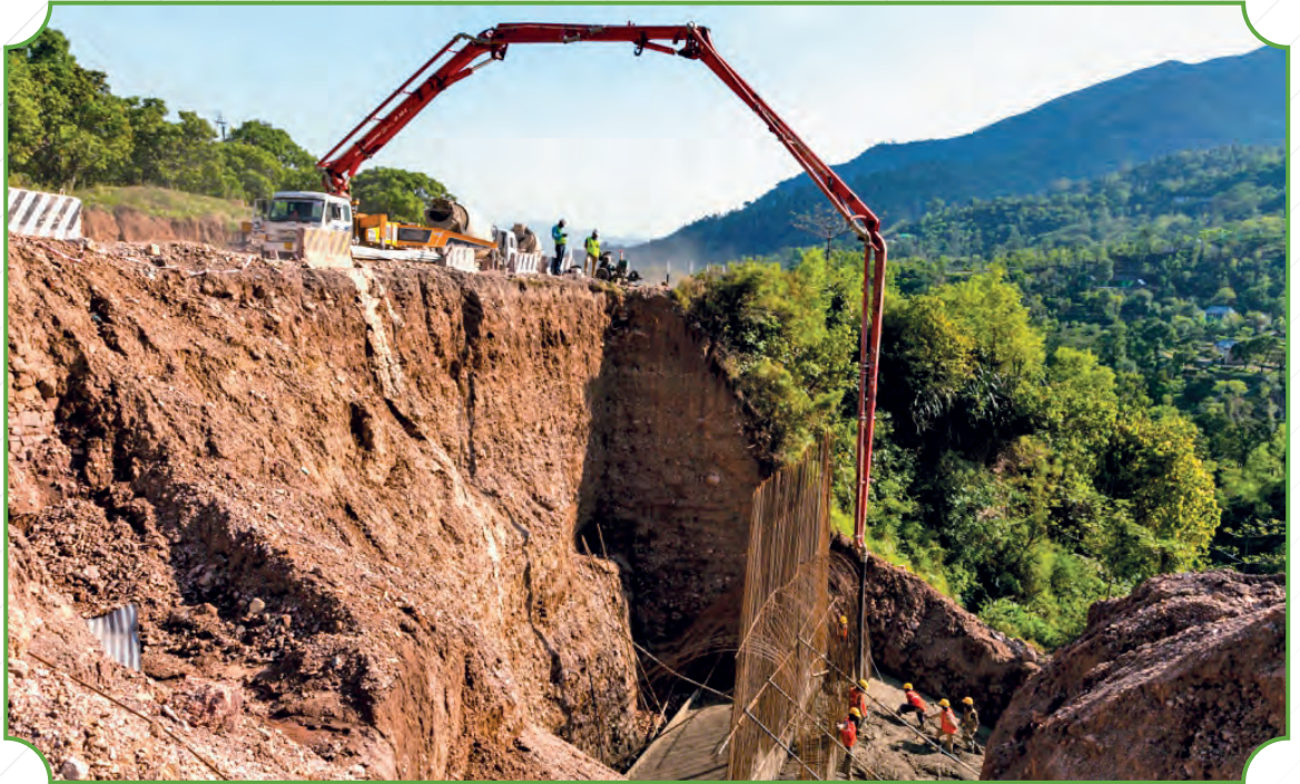
Work in progress at four laning of Kiratpur Ner Chowk Section of NH-21 in Himachal Pradesh
