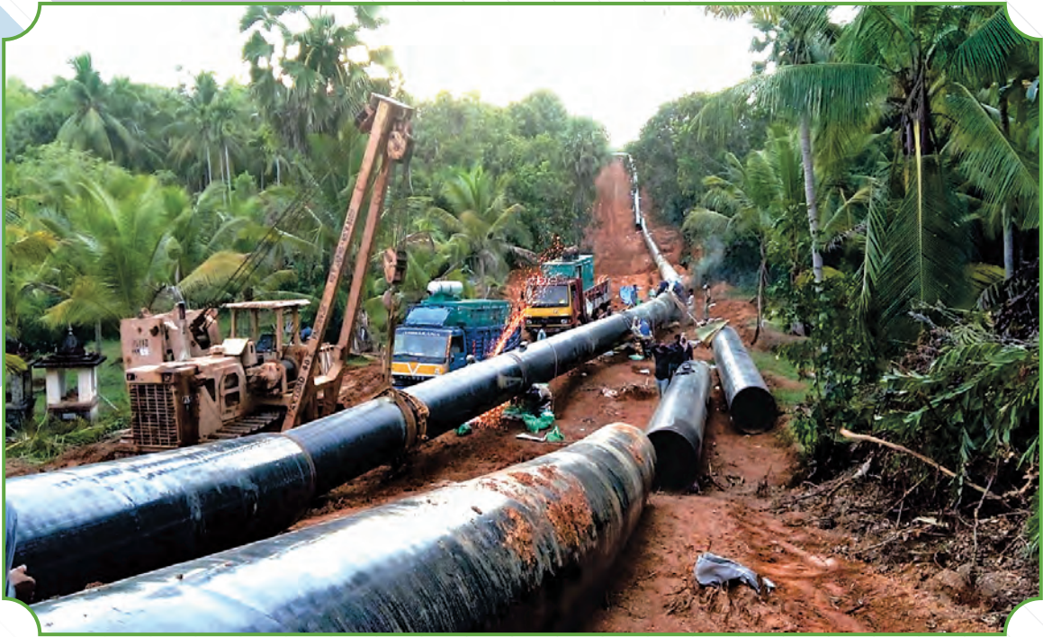
Mainline welding works for 42 inch pipeline as part of the EPC pipeline laying project for Indian Strategic Petroleum Reserves Ltd, Ministry of Petroleum & Natural Gas, Government of India in Mangalore, Karnataka
