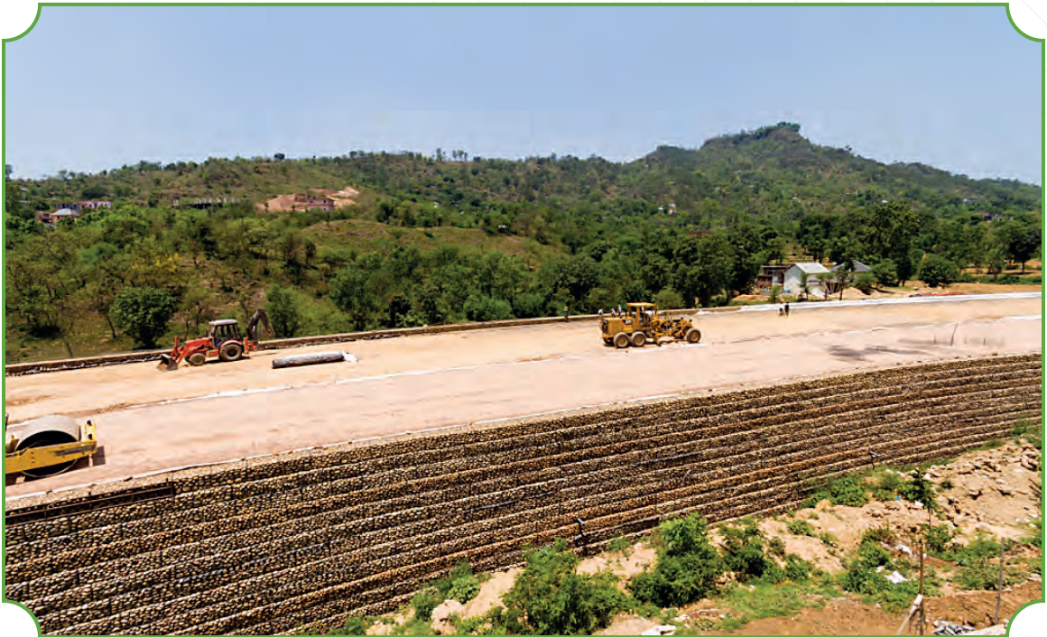
Work in progress at four laning of Kiratpur Ner Chowk Section of NH-21 in Himachal Pradesh
