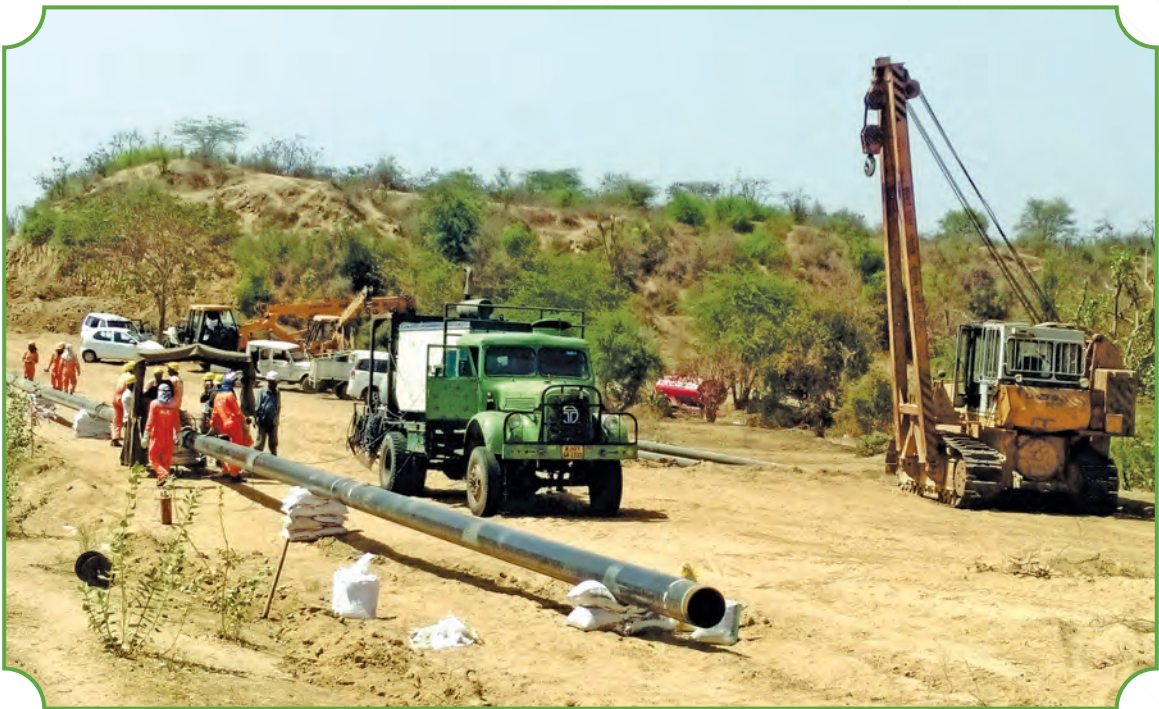
Mainline welding works for 12 inch pipeline in progress for natural gas pipeline project of Gas Authority of India Limited (GAIL) in Gujarat
