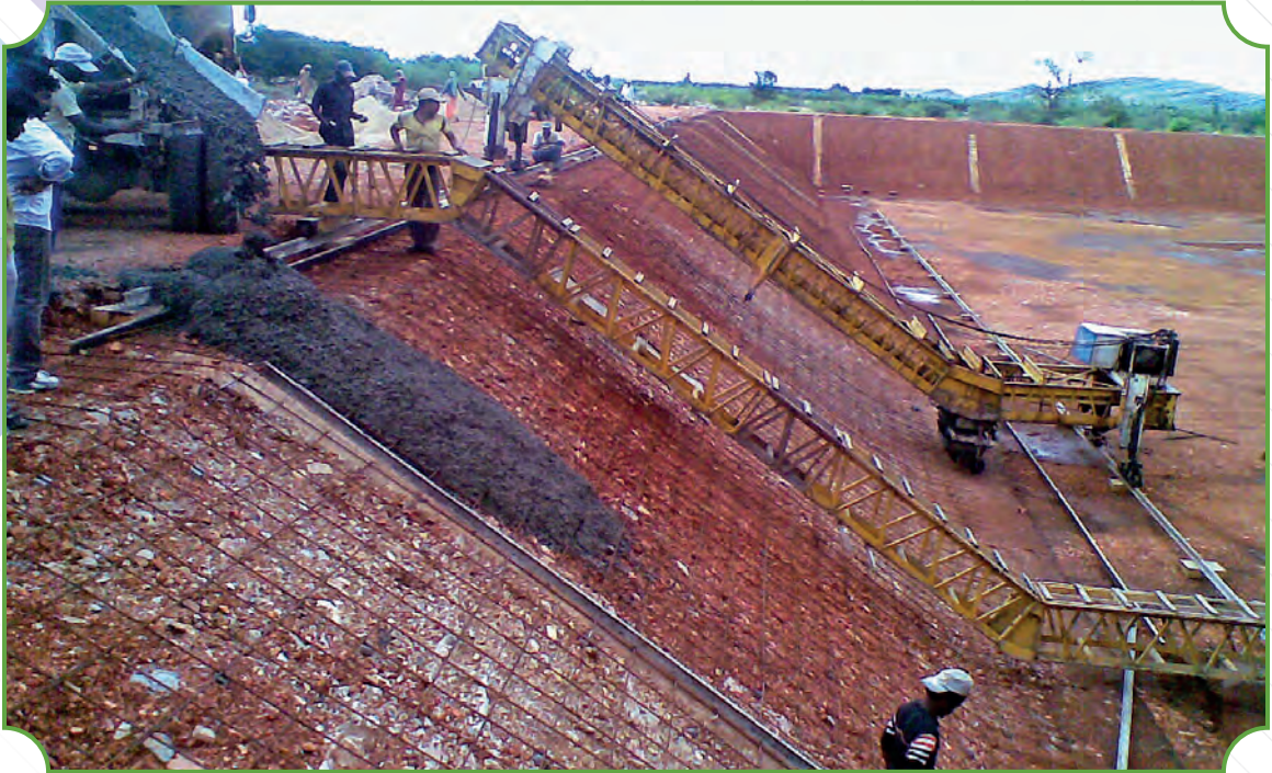
CC lining work in progress at main canal as part of Lingala irrigation project in Kadapa district of Andhra Pradesh
