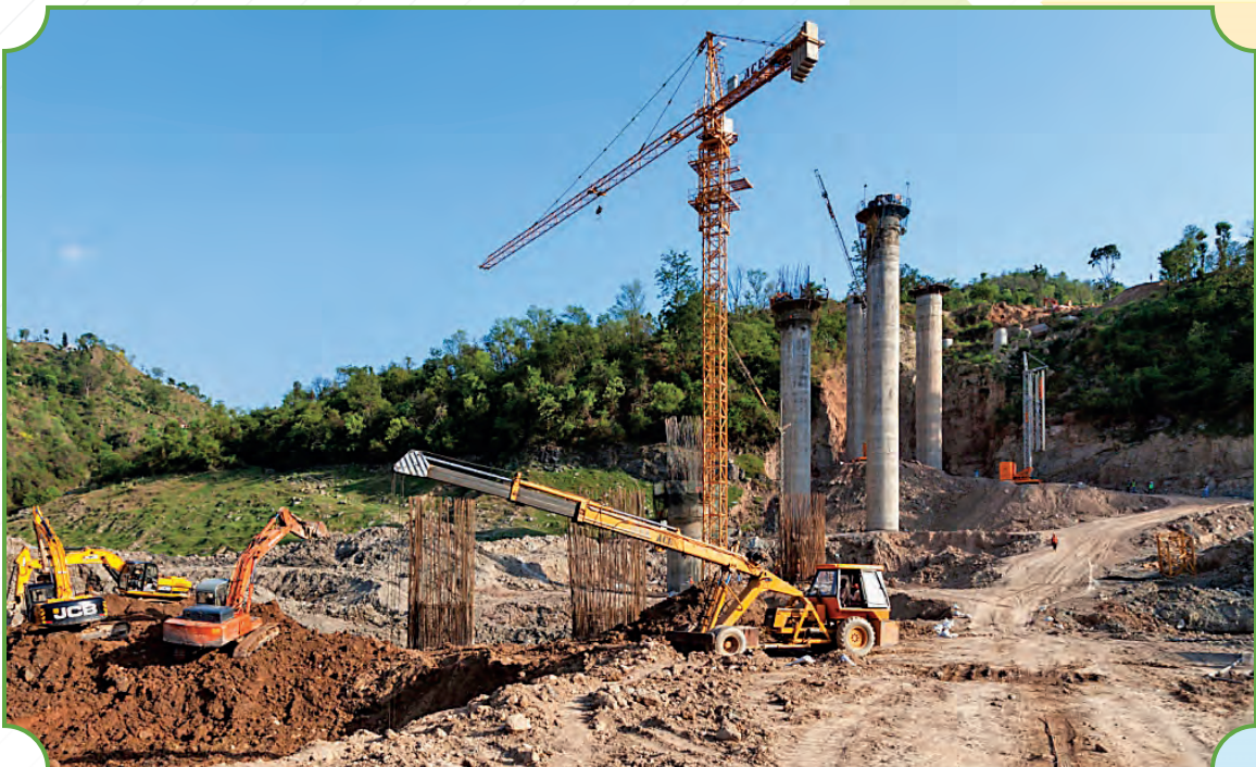
Work in progress at four laning of Kiratpur Ner Chowk Section of NH-21 in Himachal Pradesh
