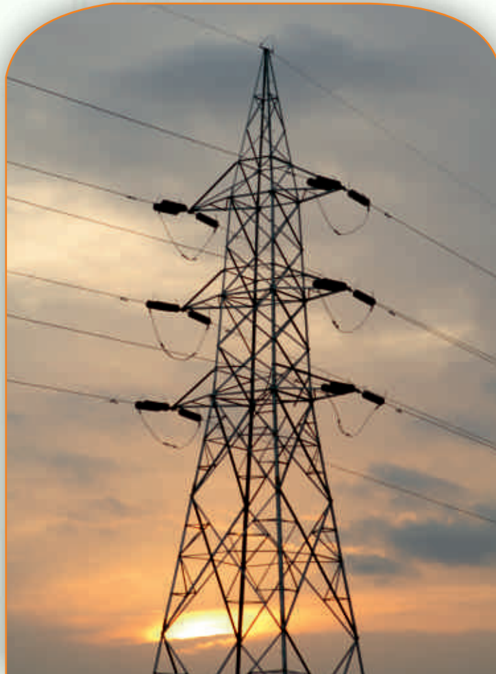
Transmission Line at Hubli for Karnataka Power Transmission Corporation Limited.
