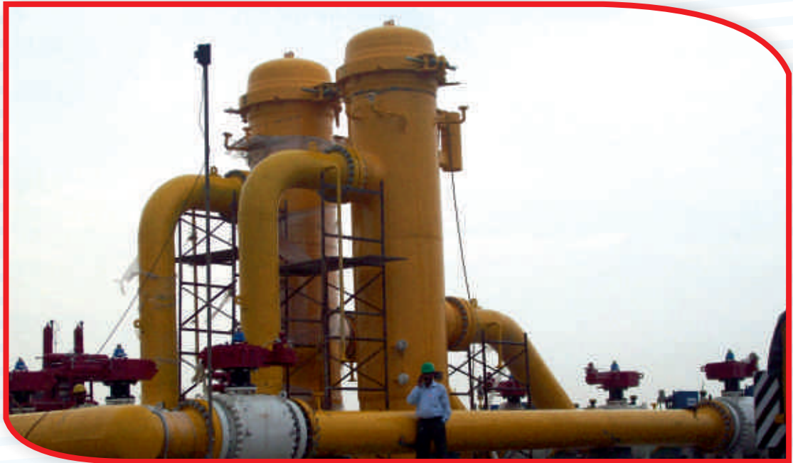
Asia's largest metering Skid erected by Maytas Infra Limited at Jamnagar in record time
